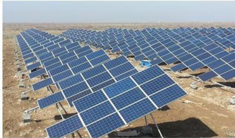
FIGURE 5 DECENTRALIZED SOLAR TRACKER
